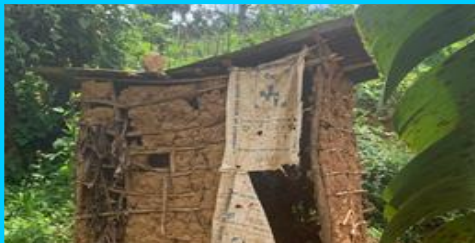
The dilapidated Toilet structure that was used by the community at Kinyarushengye
